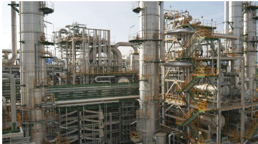
Illustration 2. Picture of a modern refinery showing all the various separation, upgrading, and conversion processes and piping.
